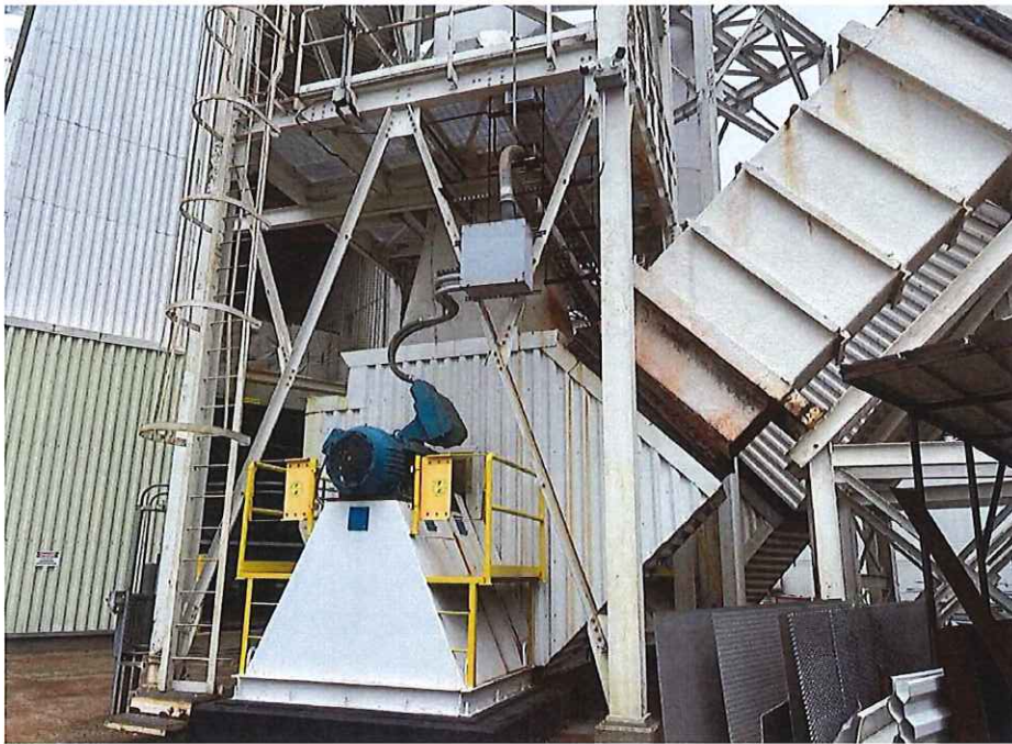
Induced Draft Fan
